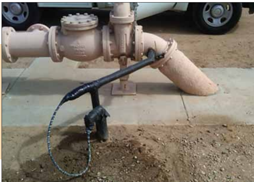
During the final injection cycles of the demonstration project, an insulated feed line was used to introduce sodium metabisulfite into the injected water to remove chlorine residual and eliminate trihalomethane formation potential.
